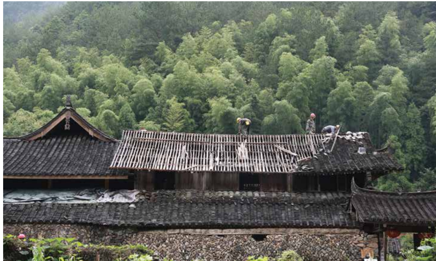
Restoration of an old house in the village. Photo by San Jin 徐岙底村古建筑修缮 摄影:三金
