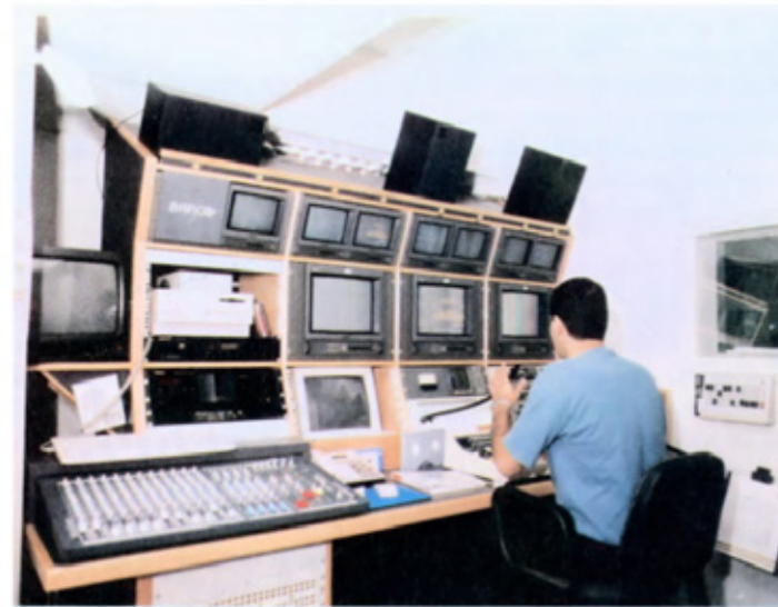
The control room of the Open University of Israel's satellite studio.
